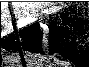
Concrete weir and pond leveler controlling water levels at the outflow of the wetland area on the west boundary of the Coats Marsh RP. (FBER Ltd photo)
