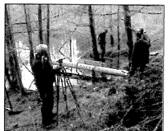
Installation of Clemson Pond Leveler in October 2009 by RDN and TNT staff (RDN photo)
