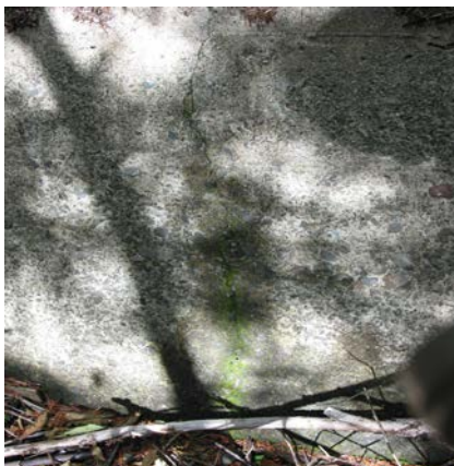
29 - Saddle Dam – Crack Closeup
