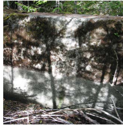
28 - Saddle Dam – Old Crack
