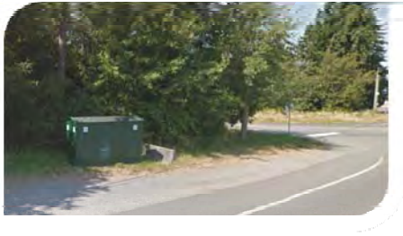
Ware Road Pressure Reducing Valve (2000)
