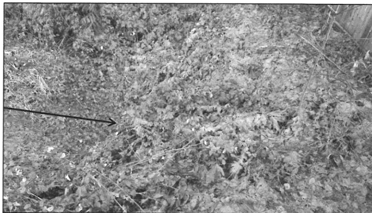
Photo 2. The upstream end of the culvert is approximately 5m from the parcel boundary
