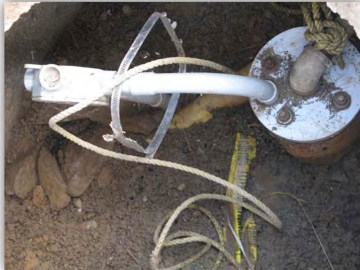
Rollo McClay Wellhead Close-up in 2012
