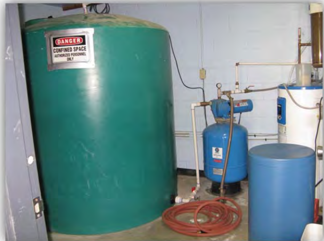
Rollo McClay Water Cistern
