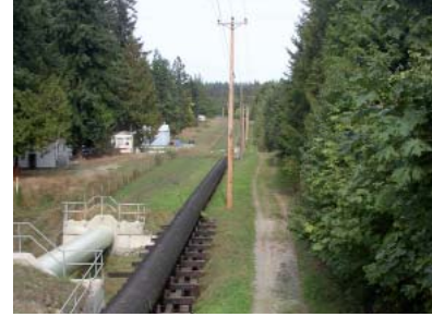
The Harmac Pipeline is a continuous utility corridor cutting through the centre of EAA that is not publicly accessible at present, but should be monitored for long-term opportunities for public access.
