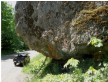
Photo 13. The Horne Lake Main on the west side of the lake traverses a slide area.
