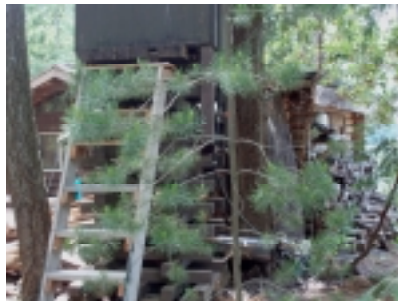
Photo 35. Some cottages at Horne Lake are highly combustible. Flammable vegetation and ignitable materials should be removed around structures.
